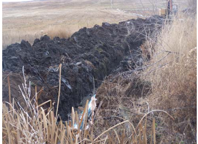
After: water will now be captured in this pipeline being installed and bypass the feedlot.
